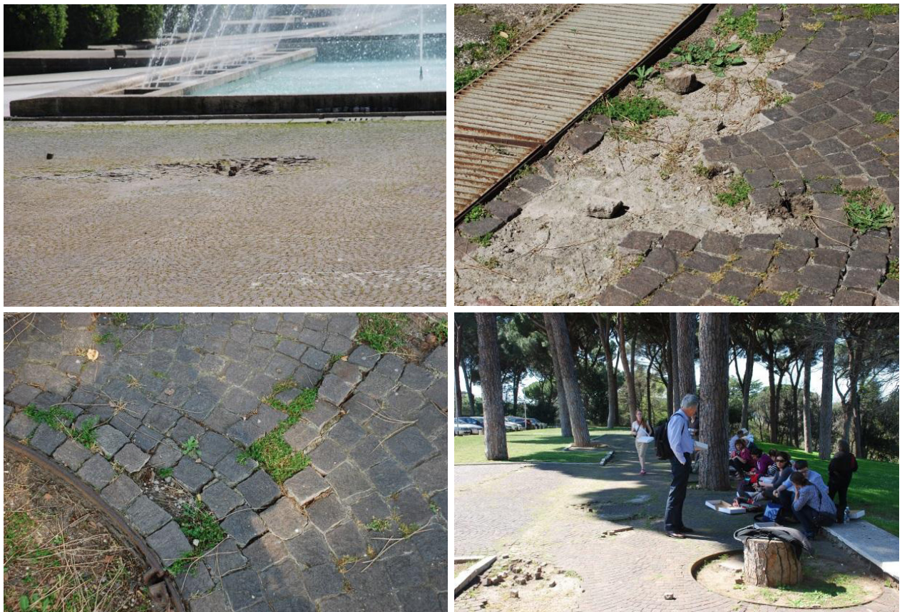
Fig. 32 (a-d) _ Technical condition of pavements in the EUR area limits the functionality and comfort for the users.
