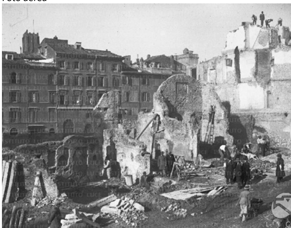
Fig. 35 _ Excavation and demolition in progress in the area of the Roman Forum, demolition of buildings in the Alexandrino district, 1932; Roma, Mediateca
